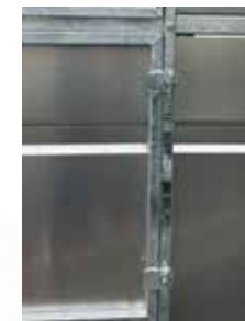
Two anti-luce pins on lower inspection door.
